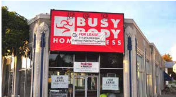
BAD DESIGN. This wall sign obscures the existing architectural features, including part of the windows, and is out of proportion to the building mass.
